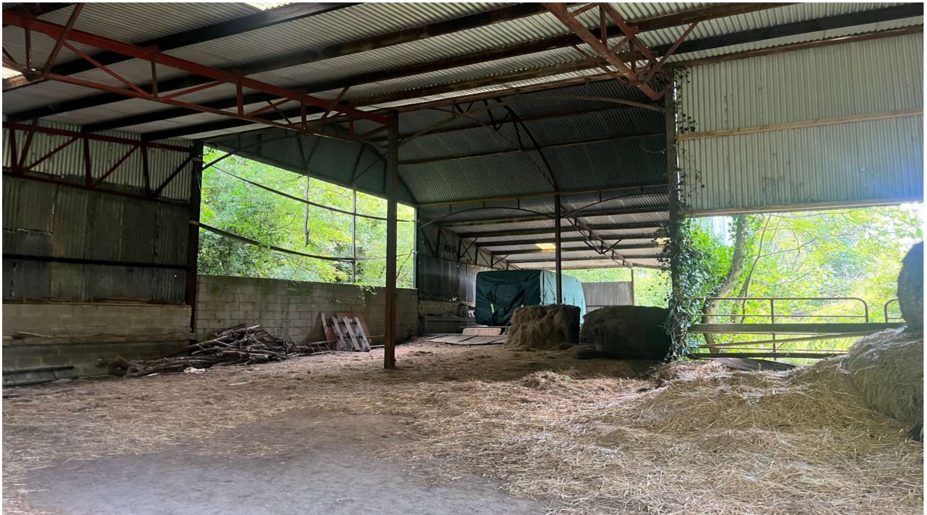
Outbuildings: Stone Bult Two Storied Farmhouse in Derelict Condition Two Span Round Roof Shed Five Span With Lean To A Number of Old Stone Outbuildings In Poor Repair
